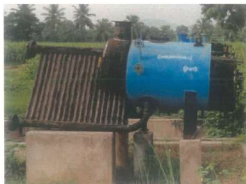
Stream Boiler (Installed at Anakapalle)
